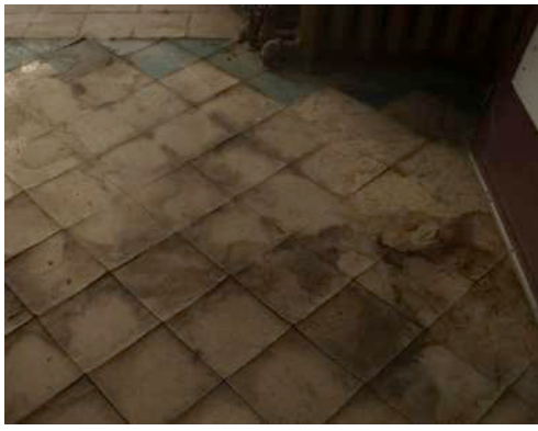
I8: Floor Tile Deterioration. Monastery of the Visitation of Holy Mary. Renée. Carleton University. 11-04-2019
