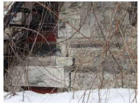
E6: Crack at Lintel. Monastery of the Visitation of Holy Mary. Tom. Carleton University. 11-04-2019
