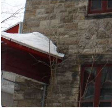
E1: Moisture Staining Elms. Monastery of the Visitation of Holy Mary. Tom. Carleton University. 11-04-2019
