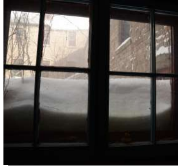
E24: Basement window snow build up. Monastery of the Visitation of Holy Mary. Tom. Carleton University. 11-04-2019
