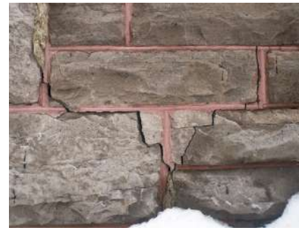
E12: Masonry Cracks. Monastery of the Visitation of Holy Mary. Renee. Carleton University. 11-04- 2019
