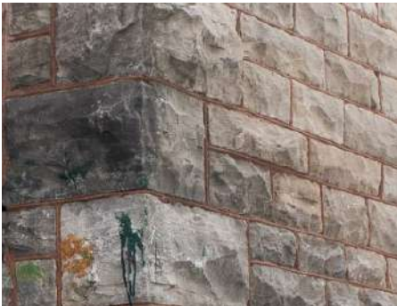
E8: Moisture Staining North Wall. Monastery of the Visitation of Holy Mary. Renee. Carleton University. 11-04-2019
