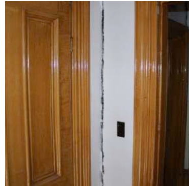
I3: Wall corner separation. Monastery of the Visitation of Holy Mary. Jason. Carleton University. 11-04-2019
