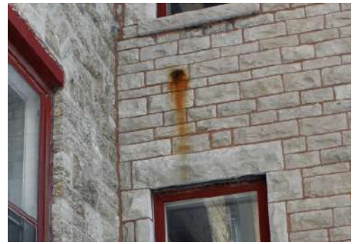
E3: Ferric Staining. Monastery of the Visitation of Holy Mary. Tom. Carleton University. 11-04-2019
