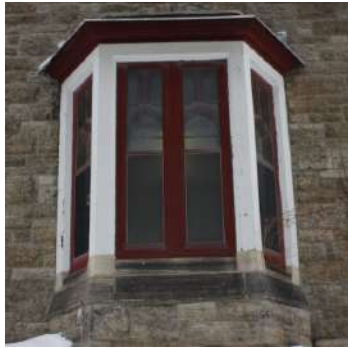
E2: Moisture Staining Elms. Monastery of the Visitation of Holy Mary. Tom. Carleton University. 11-04-2019
