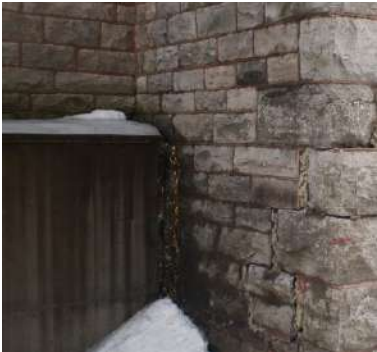
E7: Moisture Staining North Wall. Monastery of the Visitation of Holy Mary. Renee. Carleton University. 11-04-2019
