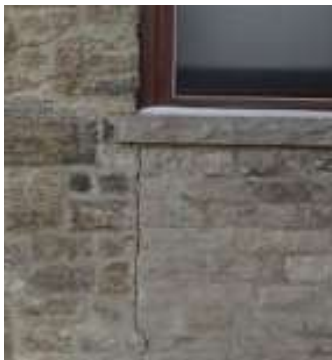
E4: Vertical Crack. Monastery of the Visitation of Holy Mary. Tom. Carleton University. 11-04-2019
