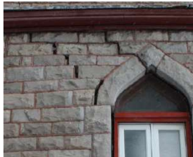
E14: Cracks near lintel. Monastery of the Visitation of Holy Mary. Jason. Carleton University. 11-04- 2019
