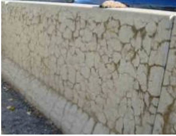
Figure: Map cracking
