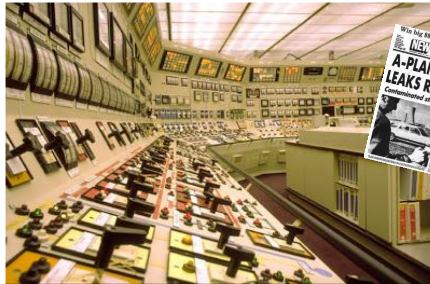
THREE MILE ISLAND CONTROL ROOM, 1979
