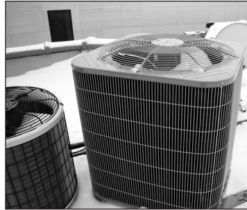
Air conditioning systems
